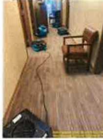
Main Level > Hallway 1 For B Offices > EQUIPMENT
