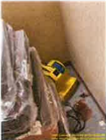
Main Level > Mechanical - B112 > EQUIPMENT
