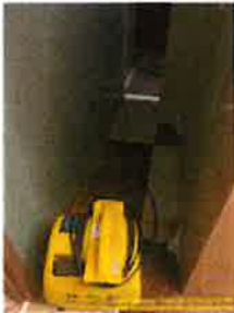
[EQUIPMENT] Work/Break Room -B110 [ Main_Level.Work/Break_Room_-B110_230620145042.jpg ]
