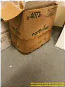
Main Level > Mechanical - B112 > BEFORE
