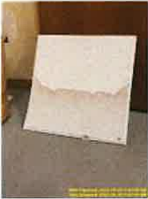
Main Level > Mechanical - B112 > BEFORE
