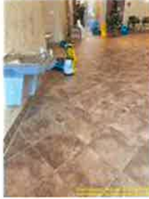
Main Level > Justice Court Lobby > EQUIPMENT
