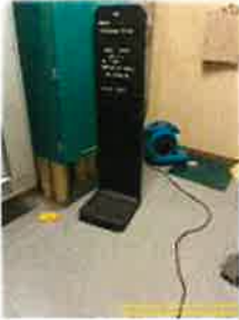
Main Level > Electrical - B111 > EQUIPMENT
