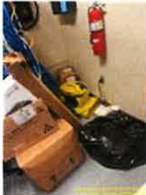
Main Level > Electrical - B111 > EQUIPMENT
