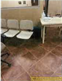
Main Level > Justice Court Lobby > EQUIPMENT
