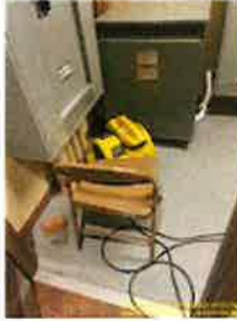
Main Level > Electrical - B111 > EQUIPMENT
